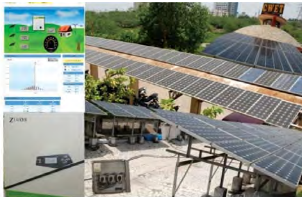
Solar PV at NIWE campus
