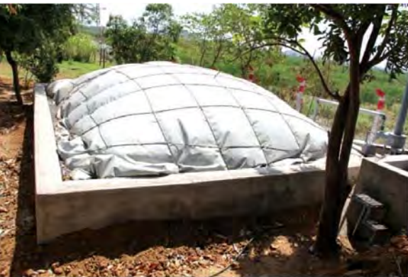
Biogas Plant at NIWE
